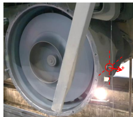
Figure 3. View of the fan during testing (view after removing the filter cover).
